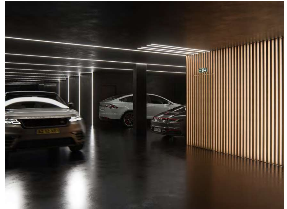
Automatically operated vehicle access door
